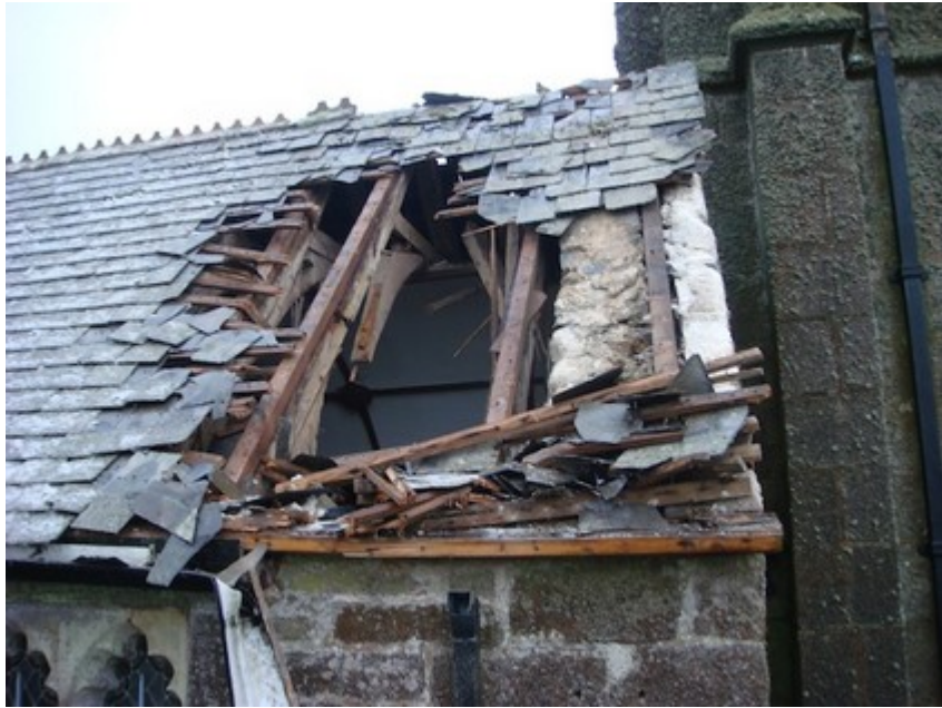
The large roof hole from outside (TR)
