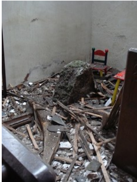
St Odulphus interior - beneath the large roof hole (RW)
