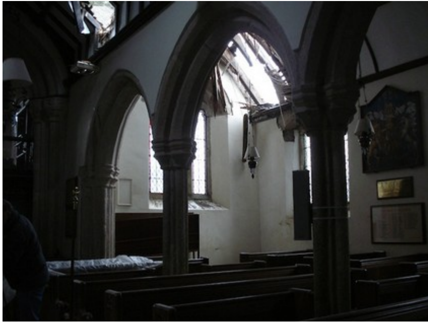
St Odulphus interior - large hole in roof (RW)
