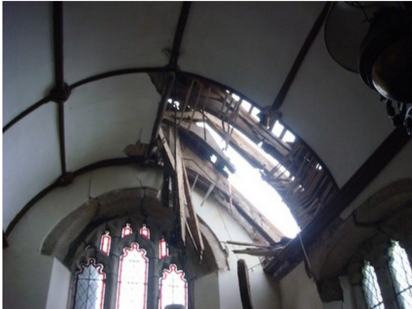
The large roof hole from inside (TR)
