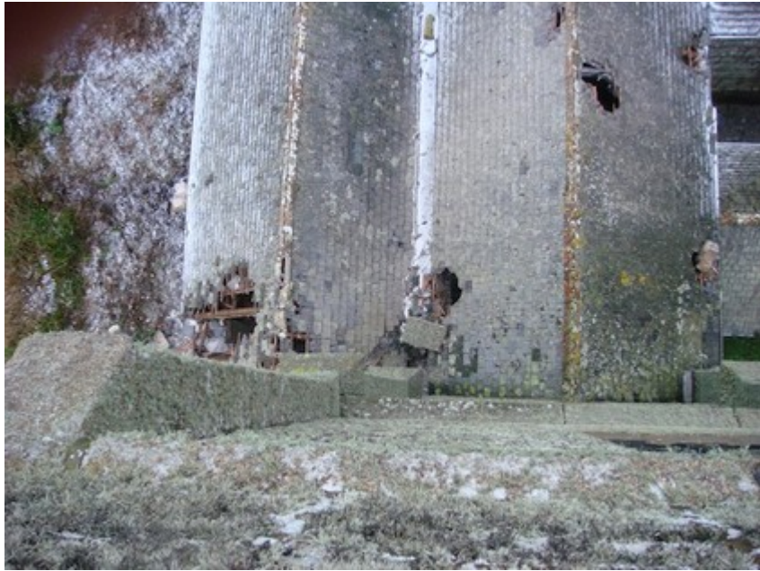
Roof holes looking down from the tower (TR)
